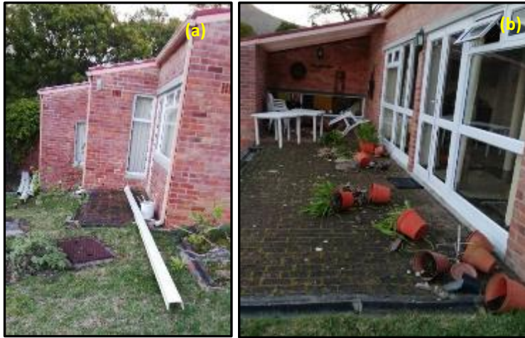
Figure 14: a) and b) damage caused by individuals at one of the houses at Ou Wingerd Road while the CT1 Troop were on their way to Groot Constantia.
